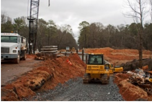
Status of Old 41 Bridge Replacement - Looking south on old 41 toward the Park.
