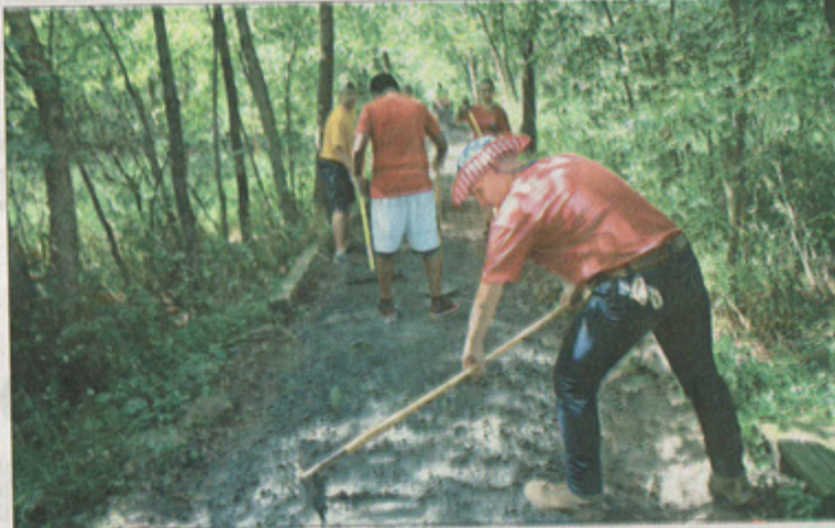
Kennesaw Mountain Trail Club members dumped crushed gravel onto the trail, and student volunteers spread it around with rakes and shovels. / Ross Williams
